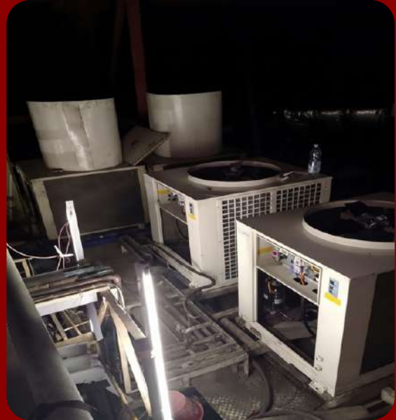
Instalasi AC Split Duct 30 PK
